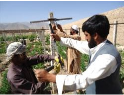
Concrete posts are shown being installed in a grape vineyard in Helmand Province.
