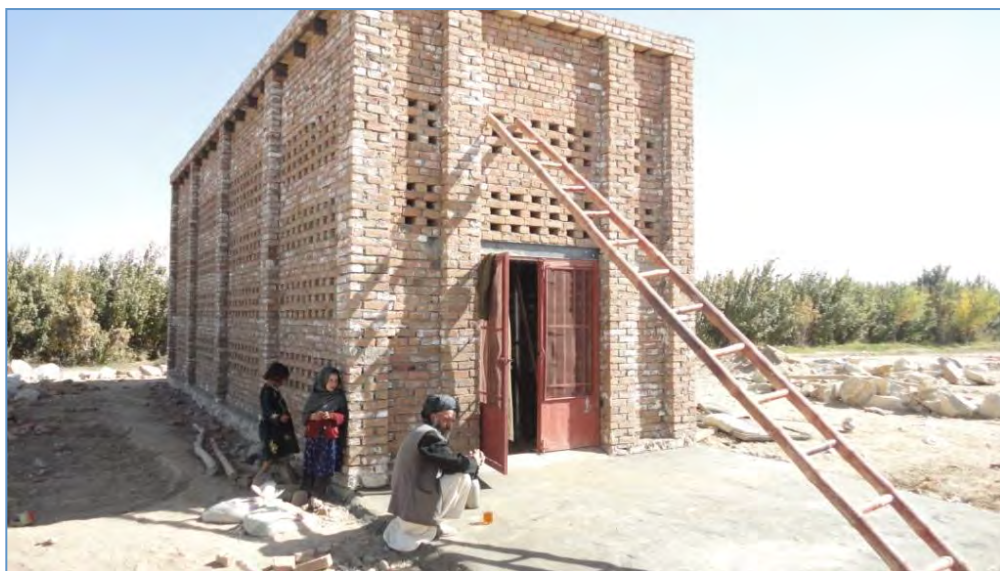
Pilot structure in Pashtun Kot, Ghazni, Afghanistan. Design improvement for next installations will extend roof eaves an additional ½ meter and extend the length from 12 to 20 meters.
